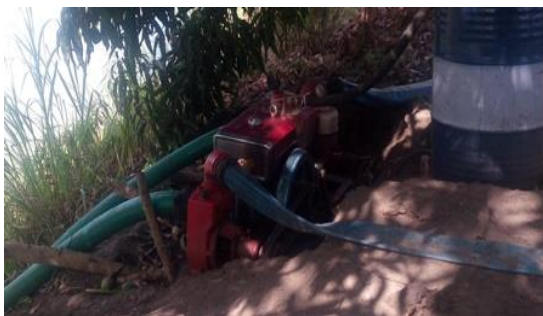
Water pump for rice irrigation financed by Mamboleo farm to farmers in Nyangala village
